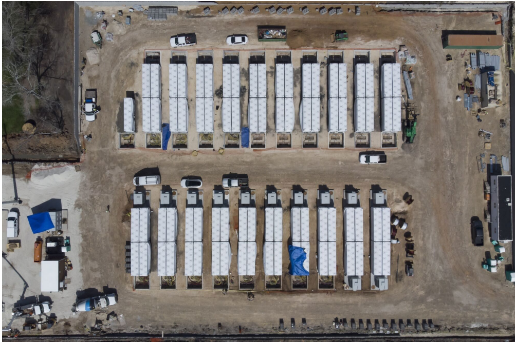
Figure. 100 MW Gambit Energy Storage Park in Angleton, Texas.
